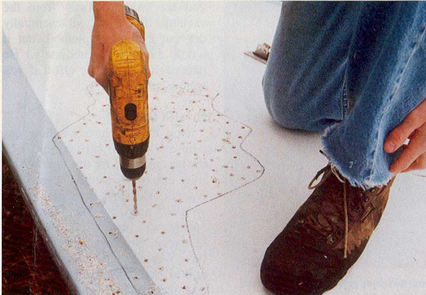
When drilling down to a wet core, but sure not to go through the bottom layer of fiberglass.
