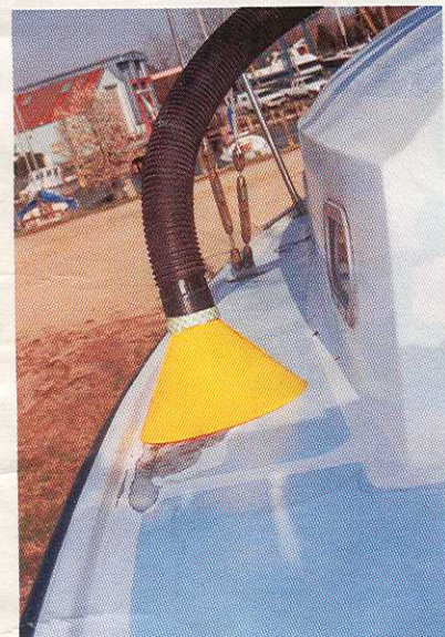
A strong vacuum will draw air between the deck drying out the space in preparation for new material.
